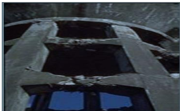
Figure 1 Bending Shear Failure in Beam
